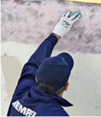
Fill along boottop
